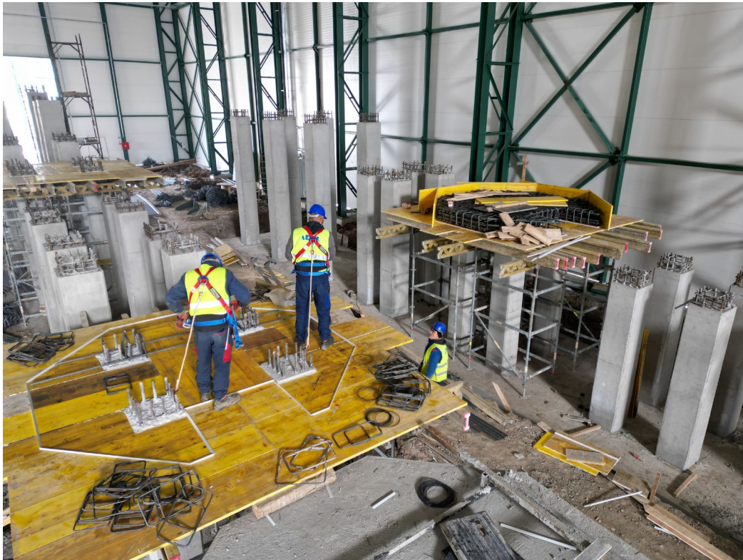
Figure 6: Inside the Vares Processing Plant
